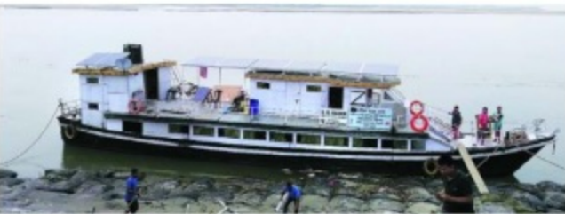
Solar power installation at Jorhat boat clinic
